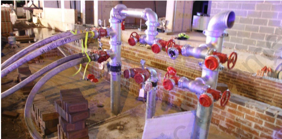
Figure 2 Lack of booster signage will cause confusion for firefighters
