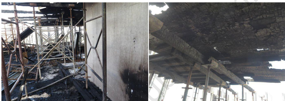
Figure 5 Damage to falsework and formwork resulting from fire
