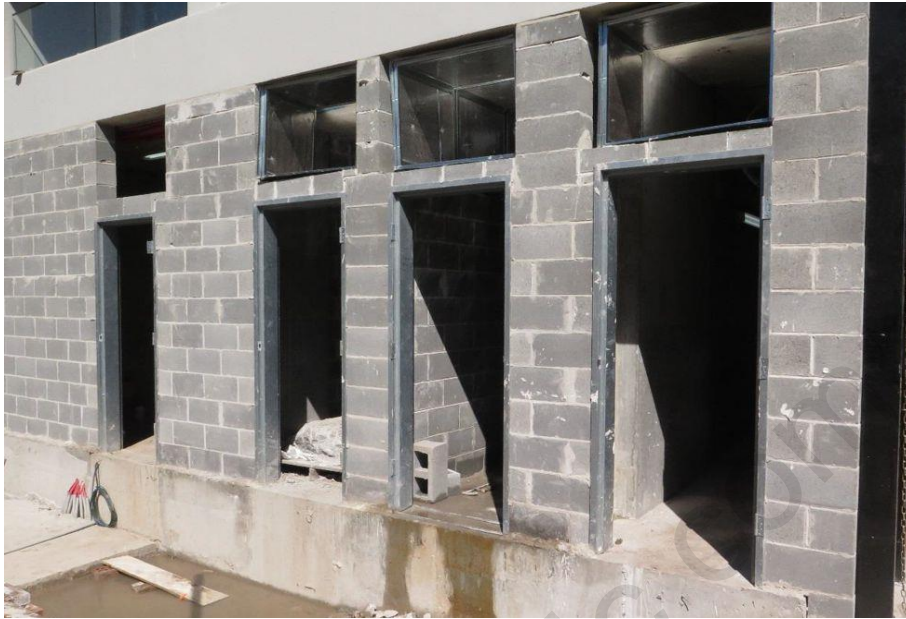
Figure 4 Doorways should identify which floors/areas they will access
